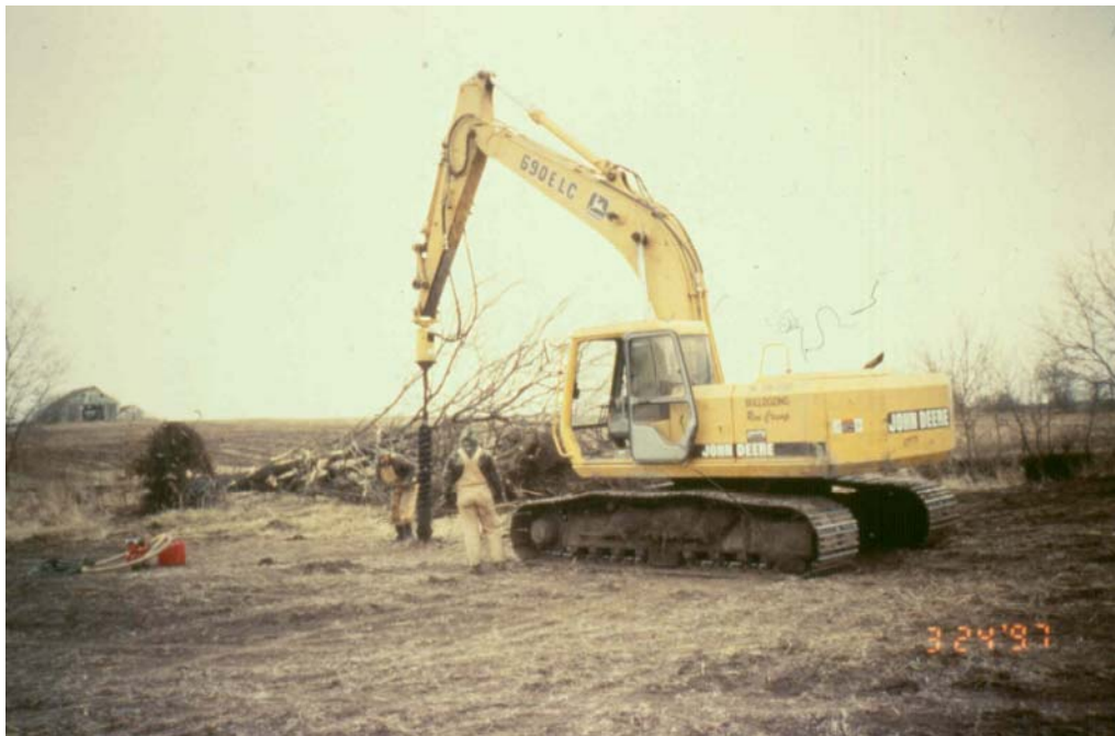
Figure 13. Track hoe and auger that was used to install dormant willow post streambank stabilization demonstration site on Money Creek in March, 1997.
